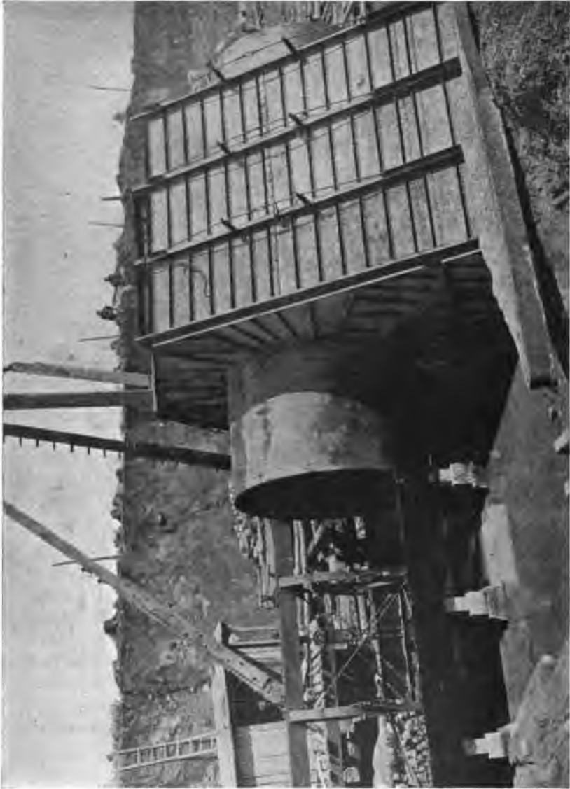
PLATE 202.—Hill View Reservoir. Steel Interior and Exterior Forms, Used for By-pass Aqueduct through Dividing Wall of Reservoir. Invert form in position on pedestal supporting carriage for moving interior forms.
